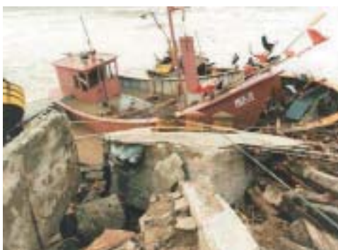
Figure 2. Damage to fishery installations in the vicinity of Międzyzdroje during the storm surge on 3 and 4 November 1995.
