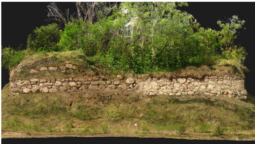
Fig. 10. Scan of the eastern wall of the tower. Graphic design: P. Domagalski.
